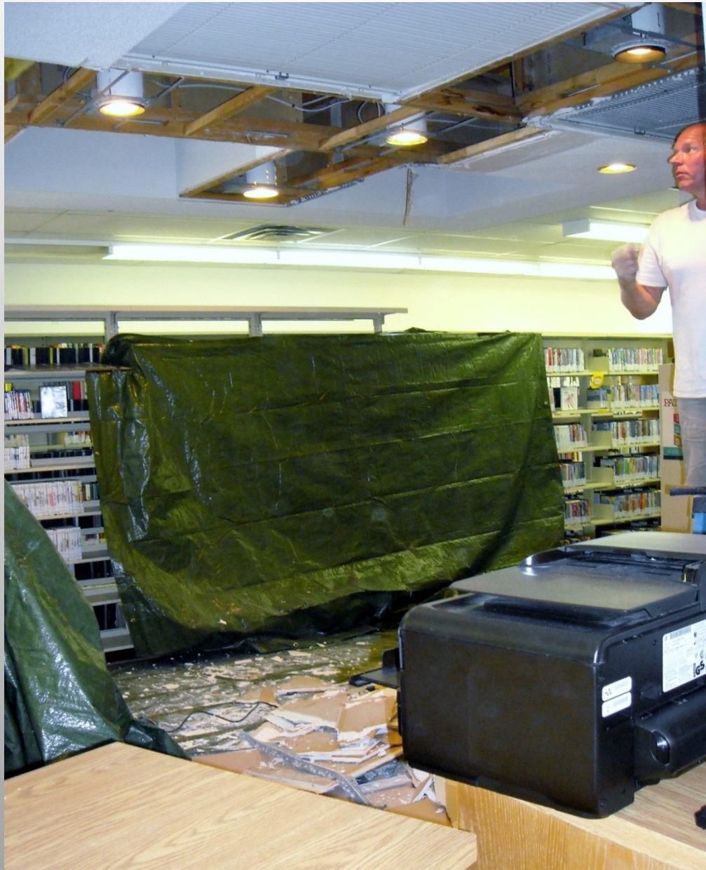
The skylight by the old circulation desk was fixed.
